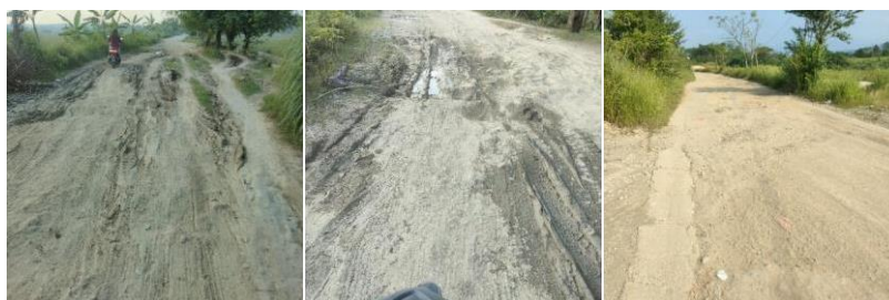
Figure 4-5. Condition of access road for the Karawang, Badami, Pangkalan,
