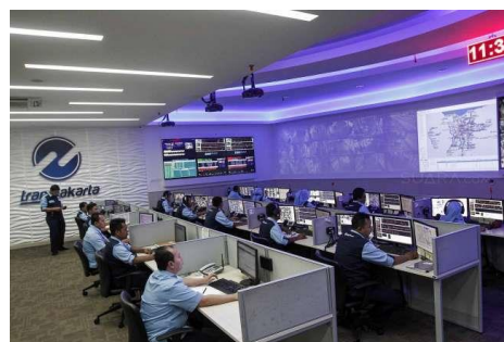
Figure 1. Command Center Room of PT Transjakarta
